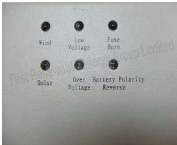
P5: LED Indicator Lights, and control button
